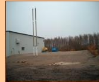
Thermosyphons to induce artificial cooling of permafrost
